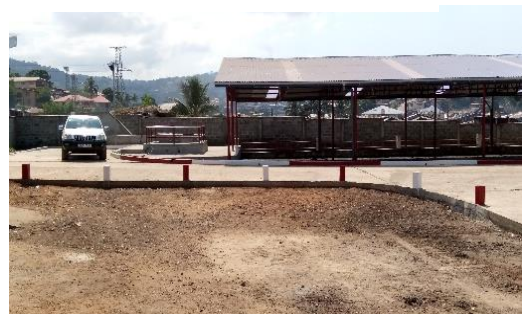
Faecal Sludge Treatment Plant, Freetown
